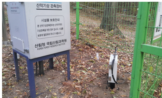
Fig. 14. The installed sensor in National institute of forest science.
